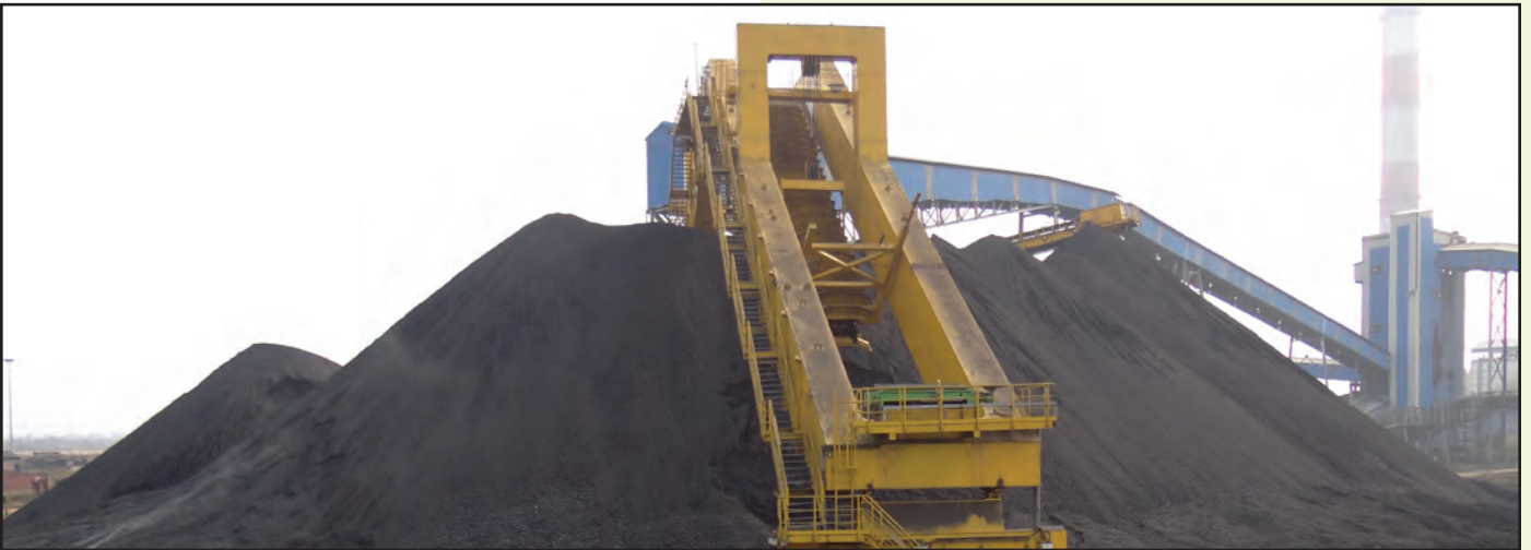
Radial Stacker Reclaimer at PP-III Bhilai
