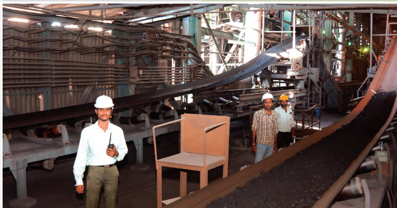
Coal Handling Plant, Bhilai PP-II (2x30 + 1x14 MW)
