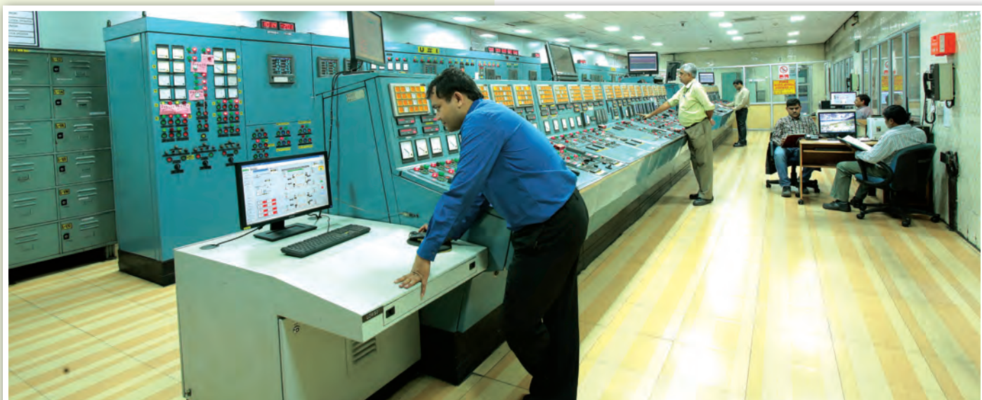
Control Room, Durgapur CPP-II
